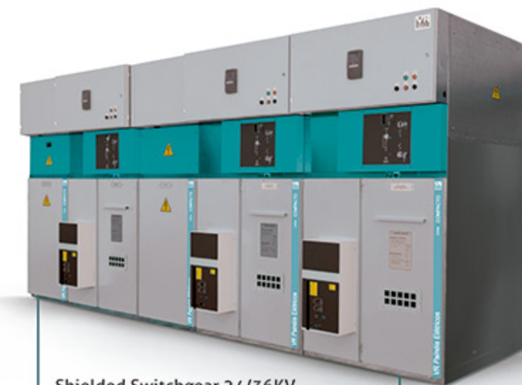
Shielded Switchgear 24/36KV tested according to technical standards
