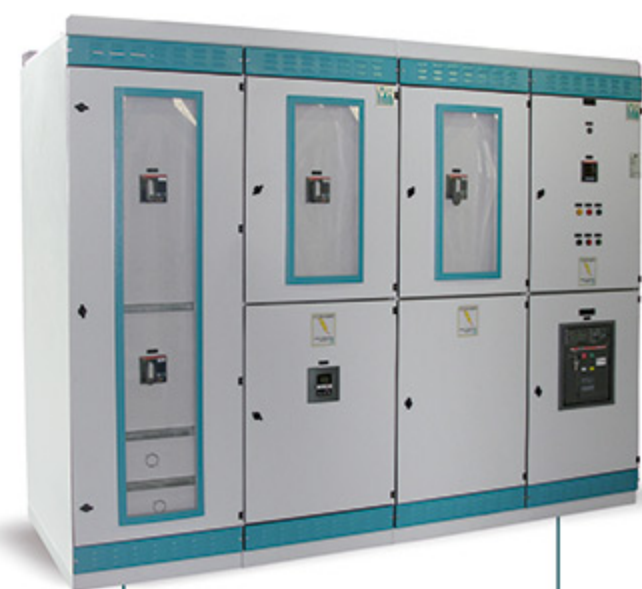
QGBT - Low-Voltage Switchboard Form 3B TTA/PTTA
