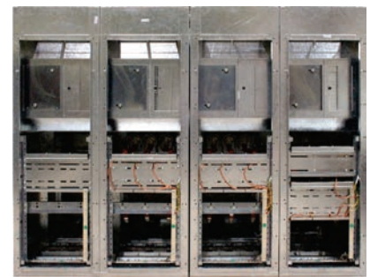
Rear view with housing of the TPs and housing of the cables and Tcs.
