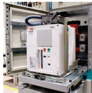
Circuit Breaker/Contactor Housing.
